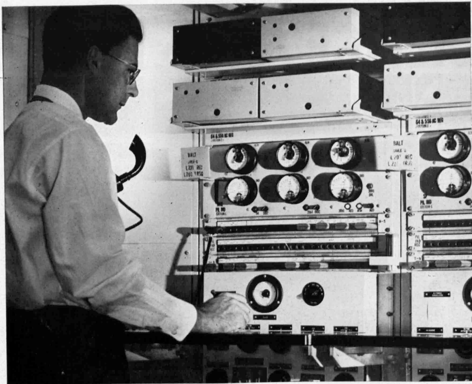
At Philadelphia, a testboard man answers as an electronic watchman calls attention to conditions on a coaxial system to Washington.
